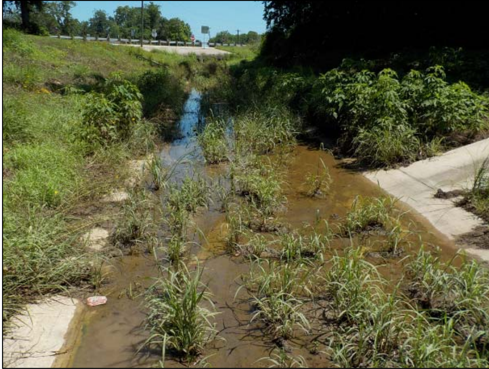
Photo 9. Another view of the northern end of Ditch 1 (north of Audubon Woods Dr), facing north (downstream).
