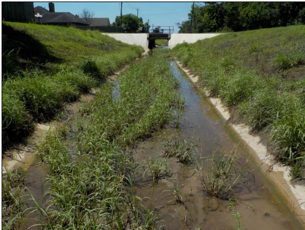
Photo 8. Another view of the northern end of Ditch 1 (north of Audubon Woods Dr), facing south (upstream).
